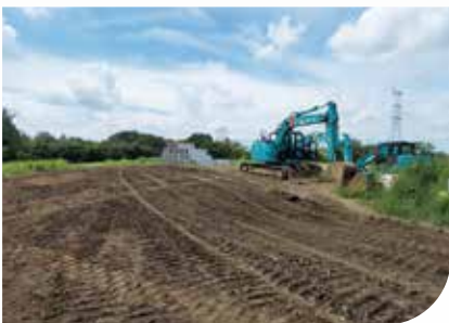
Site of Nasu Karasuyama Solar Power Plant
